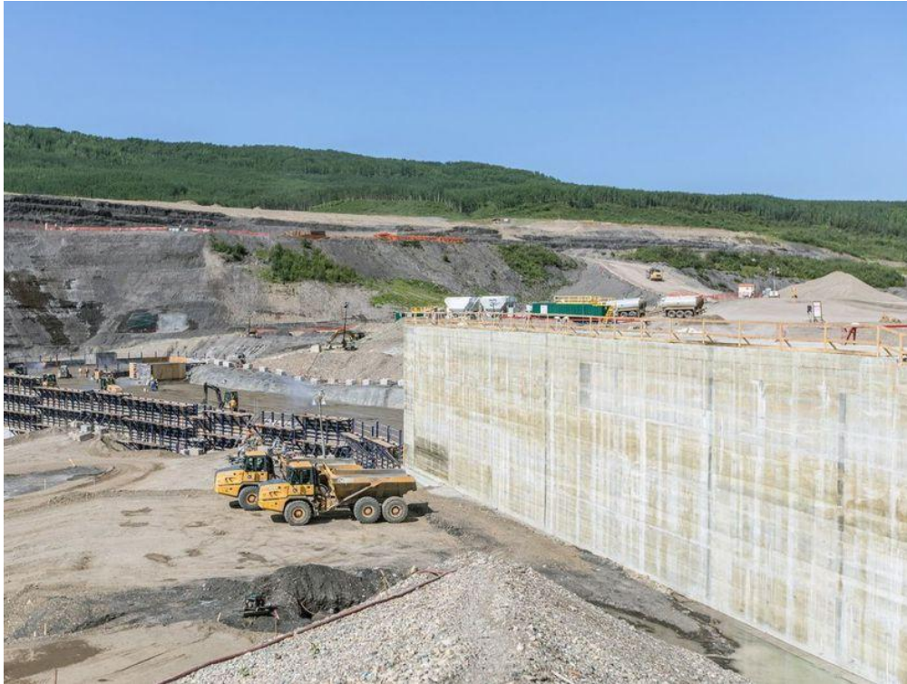
Installation of concrete for the south-bank tailrace wall in July at B.C. Hydro's Site C dam construction project on the Peace River near Fort St. John. B.C. HYDRO / PNG ADJUST
